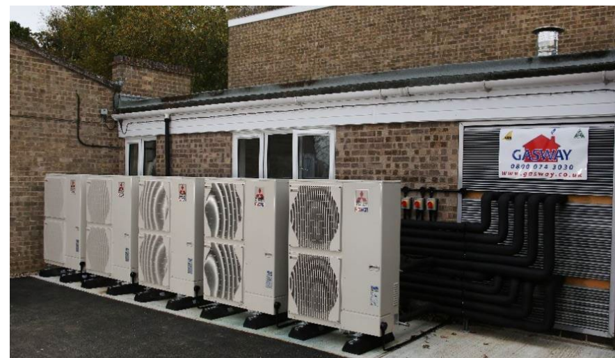
Figure 20 Air Source Heat Pump System
